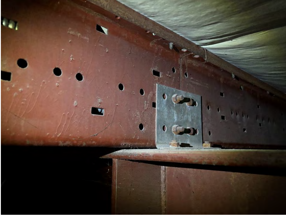
Photo 5 – Unpainted Roof Purlins in Storage Area on North Side of Arena in Excellent Condition.
