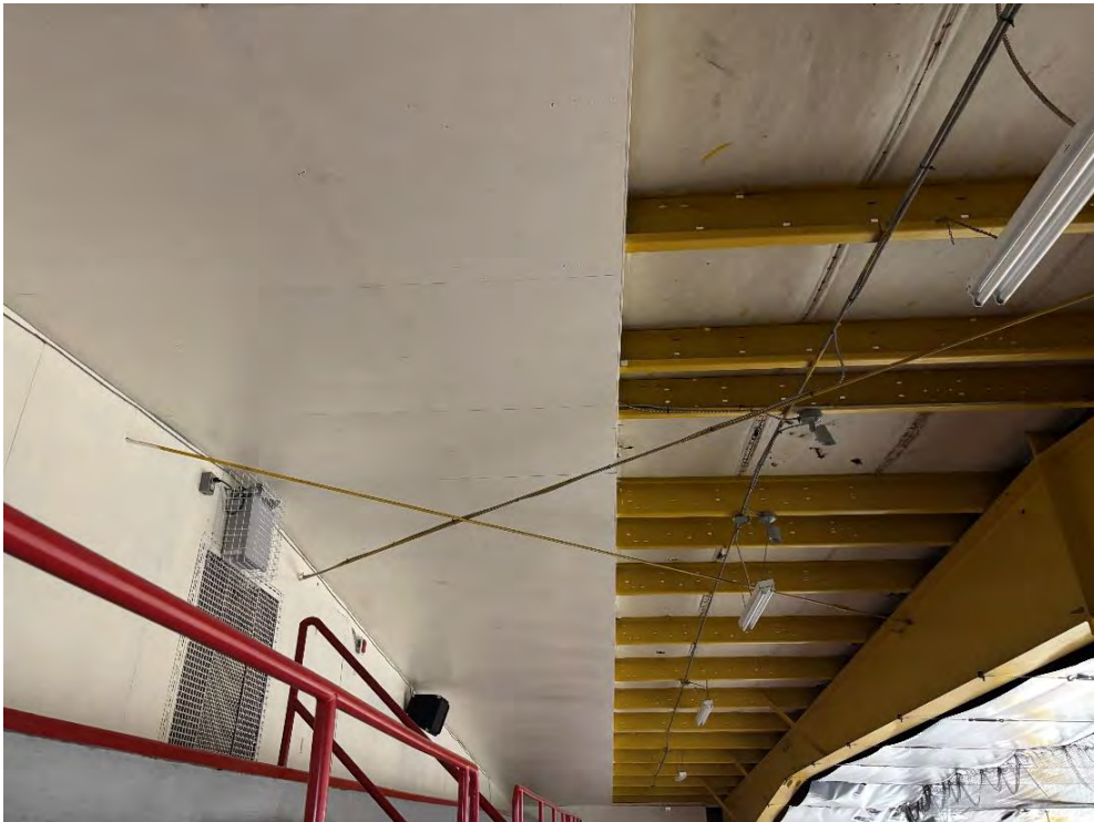
Photo 6 – Misaligned Lateral Rod Roof Bracing in Last Bay at East End of Building.
