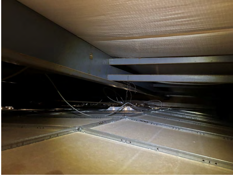
Photo 17 – Typical Roof Purlin in 1998 Addition with Two Rows of Purlin Bracing at Quarter Spans.
