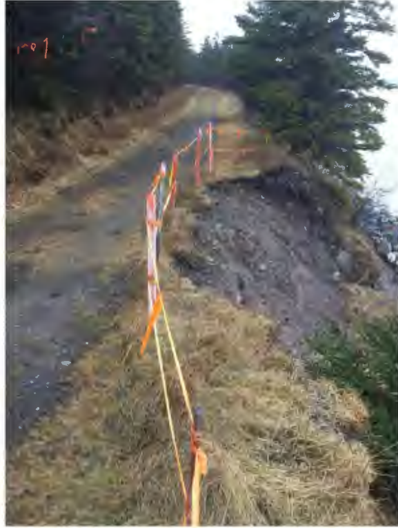
River Tillard-St. Peter's Trail Erosion (before repair)
