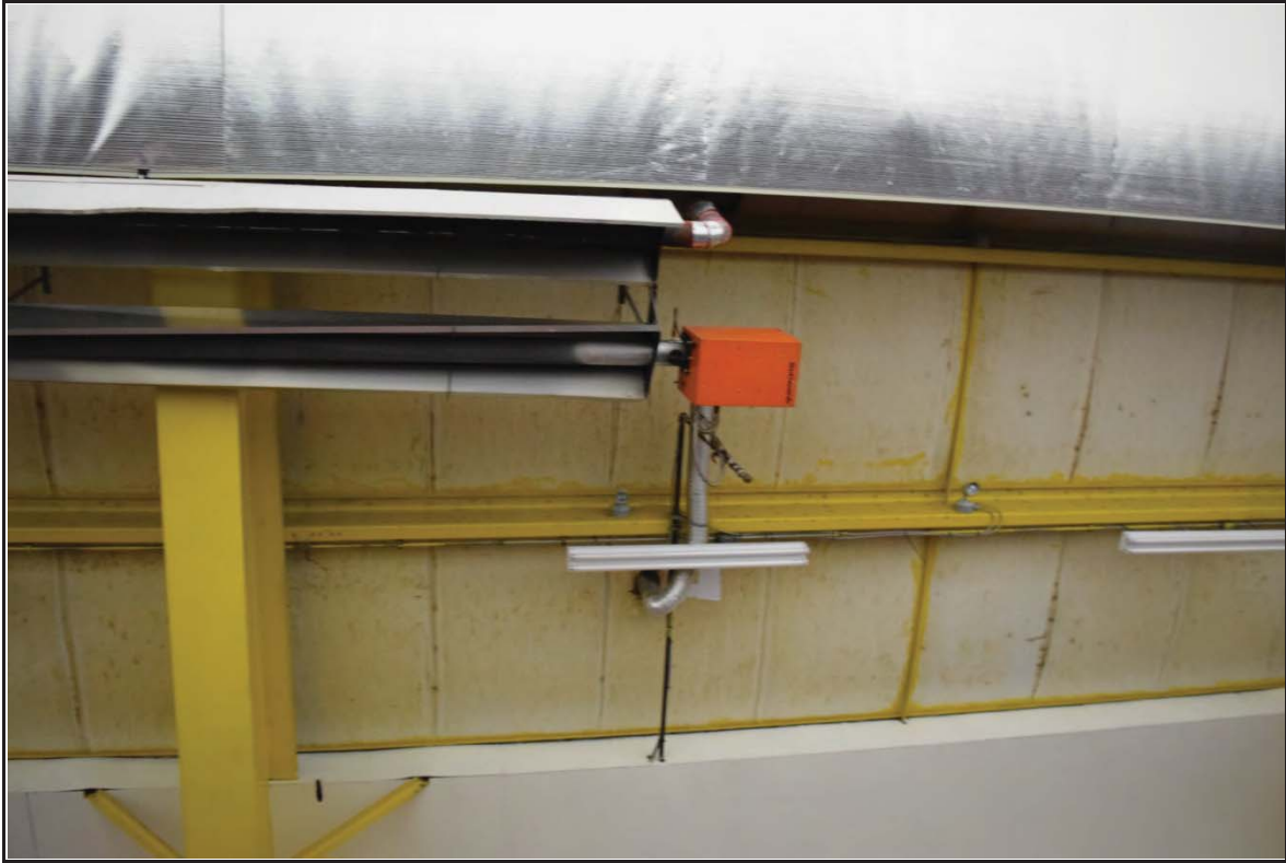
Photo 25: Typical Radiant Tube Propane Heater
