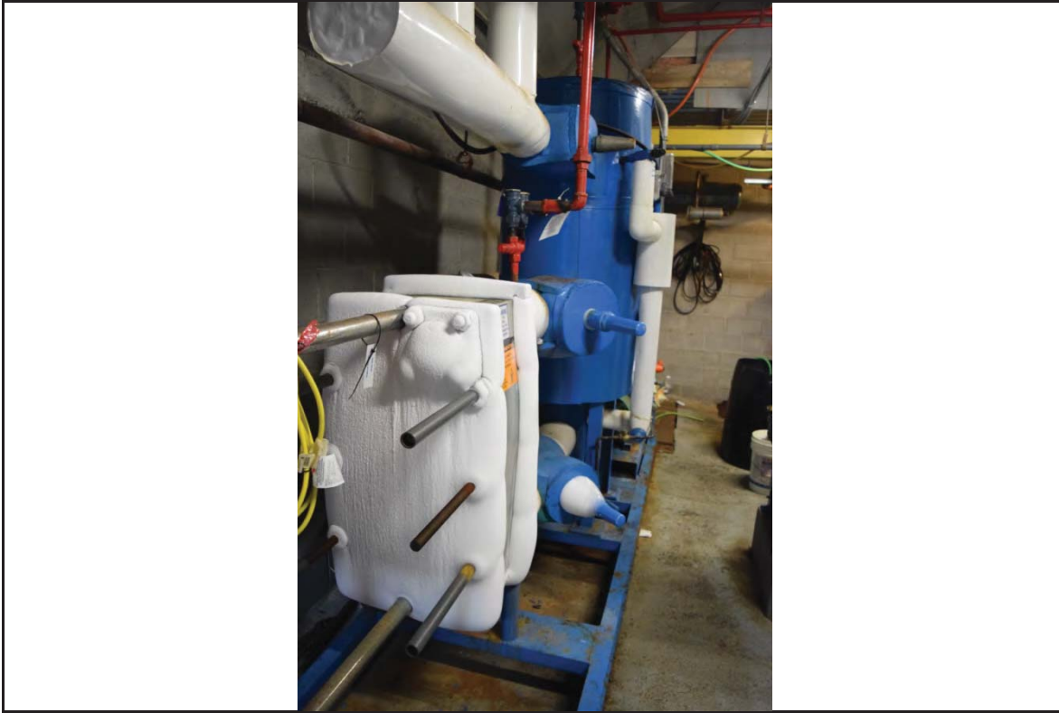
Photo 35: Skid Mounted Chiller, Vacuum Accumulator, and Brine Pump
