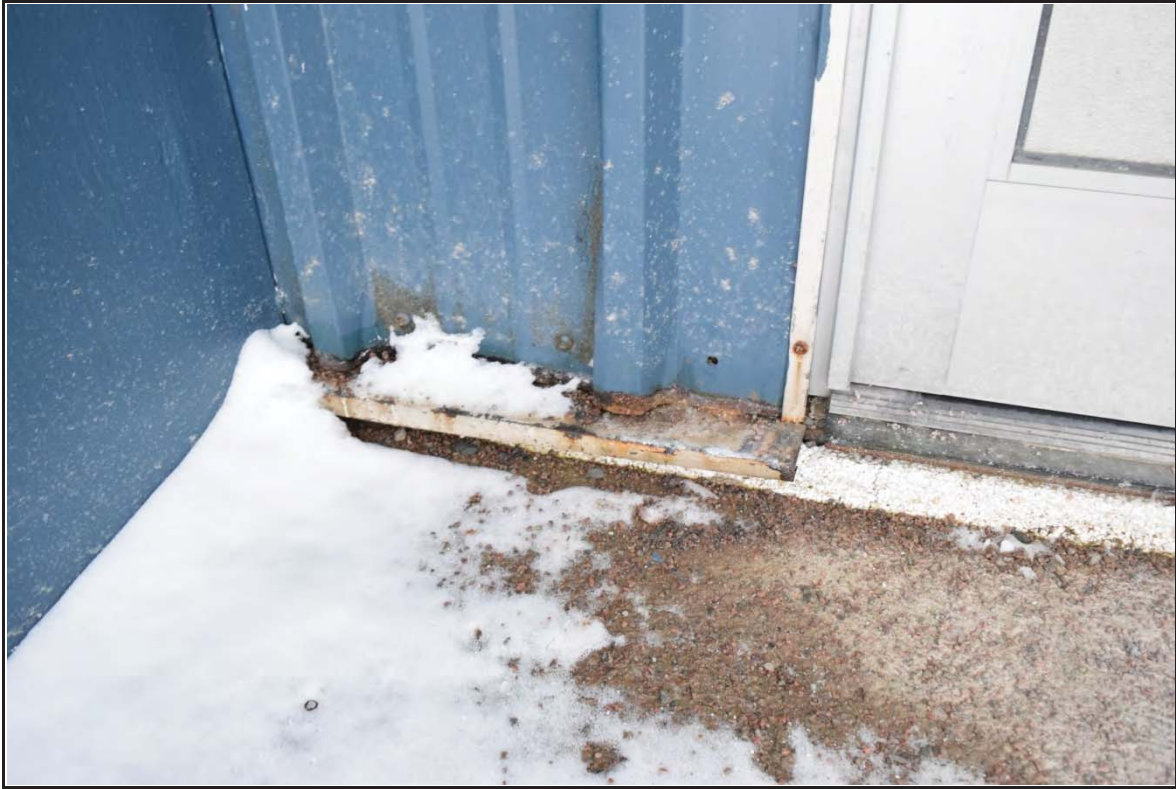
Photo 9: Corrosion at Base of Siding on North Elevation
