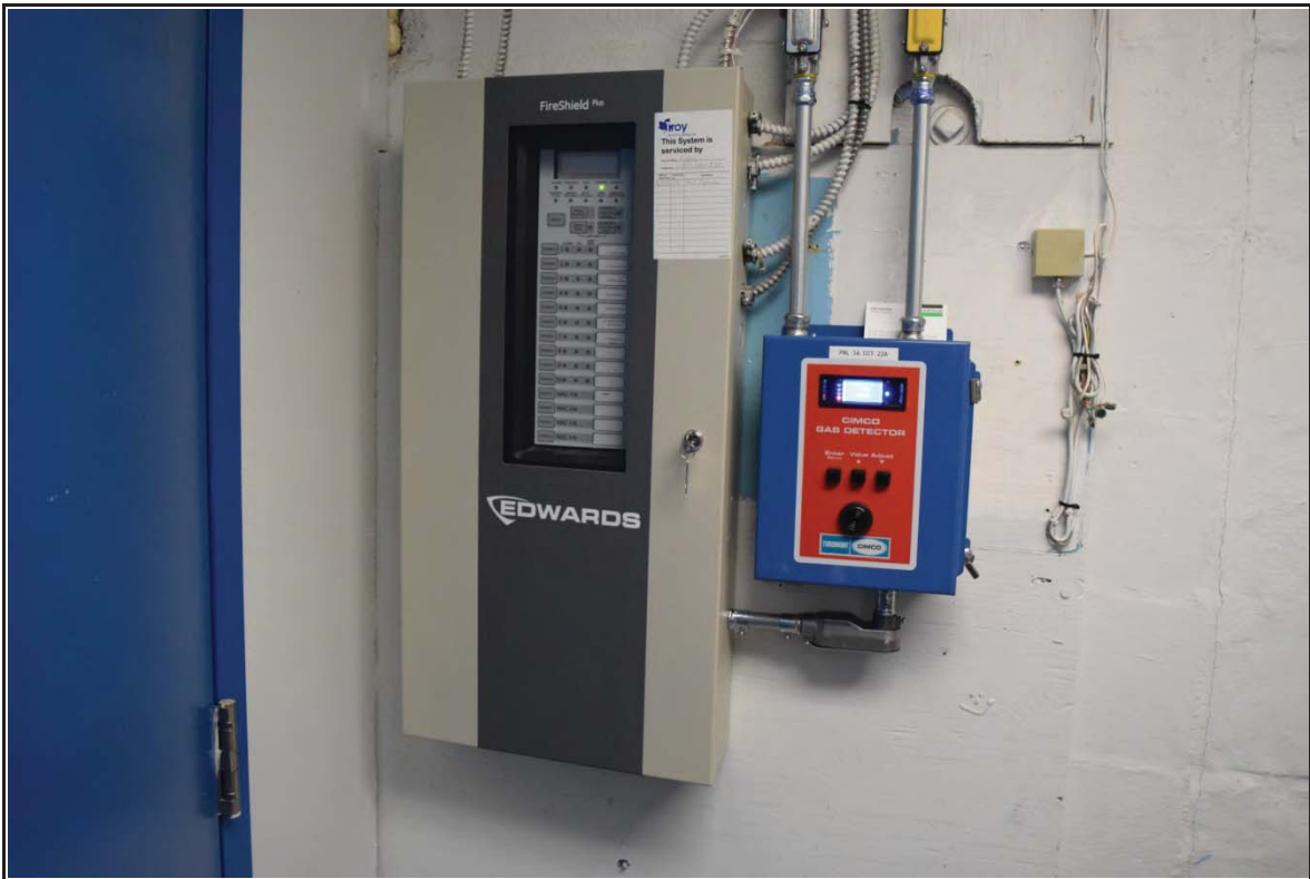
Photo 32: Edwards FireShield Plus Fire Alarm Panel, and Cimco Refrigerant Leak Alarm
