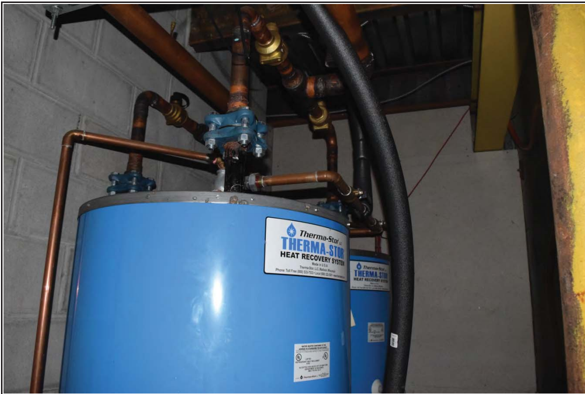
Photo 36: ThermoStor Heat Recovery Tanks
