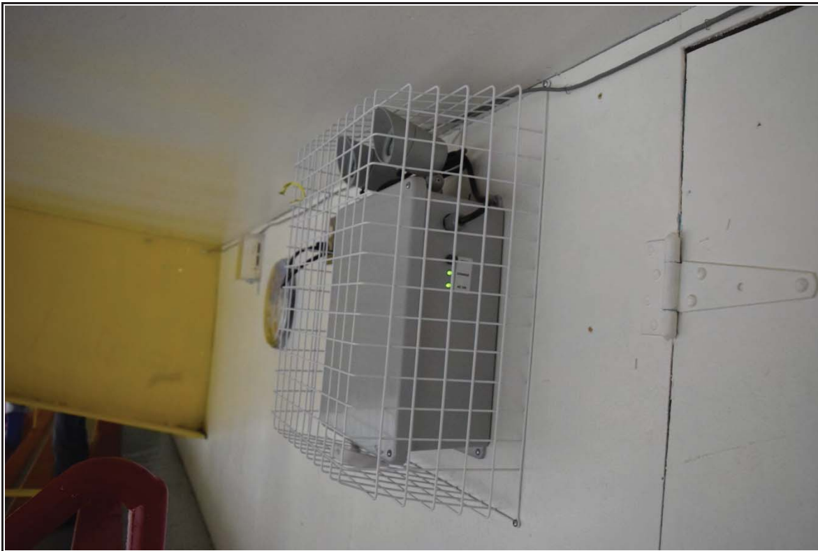
Photo 34: Typical Emergency Lighting
