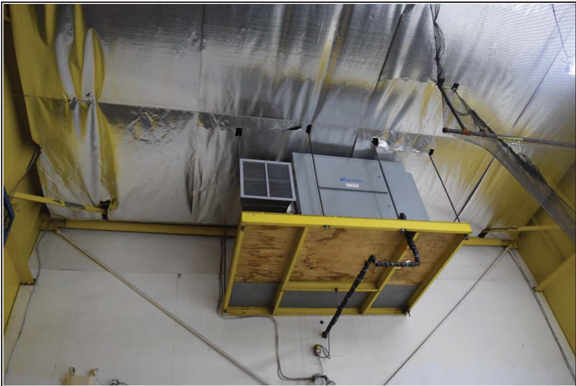
Photo 30: Eastern Dectron Dehumidifier
