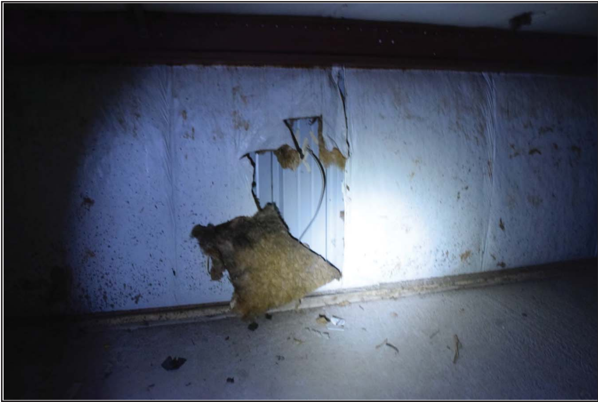
Photo 23: Damage Insulation at Upper Wall
