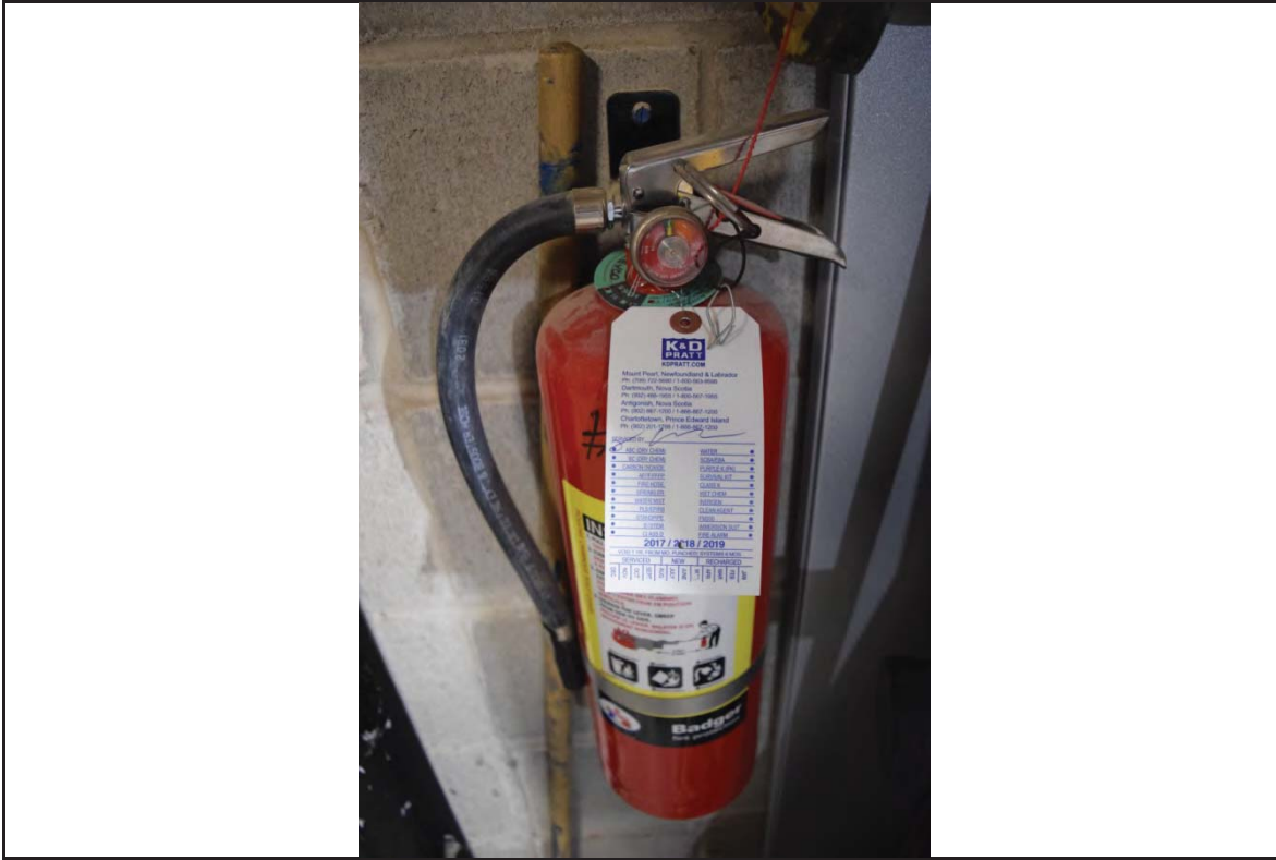
Photo 33: Typical Fire Extinguisher
