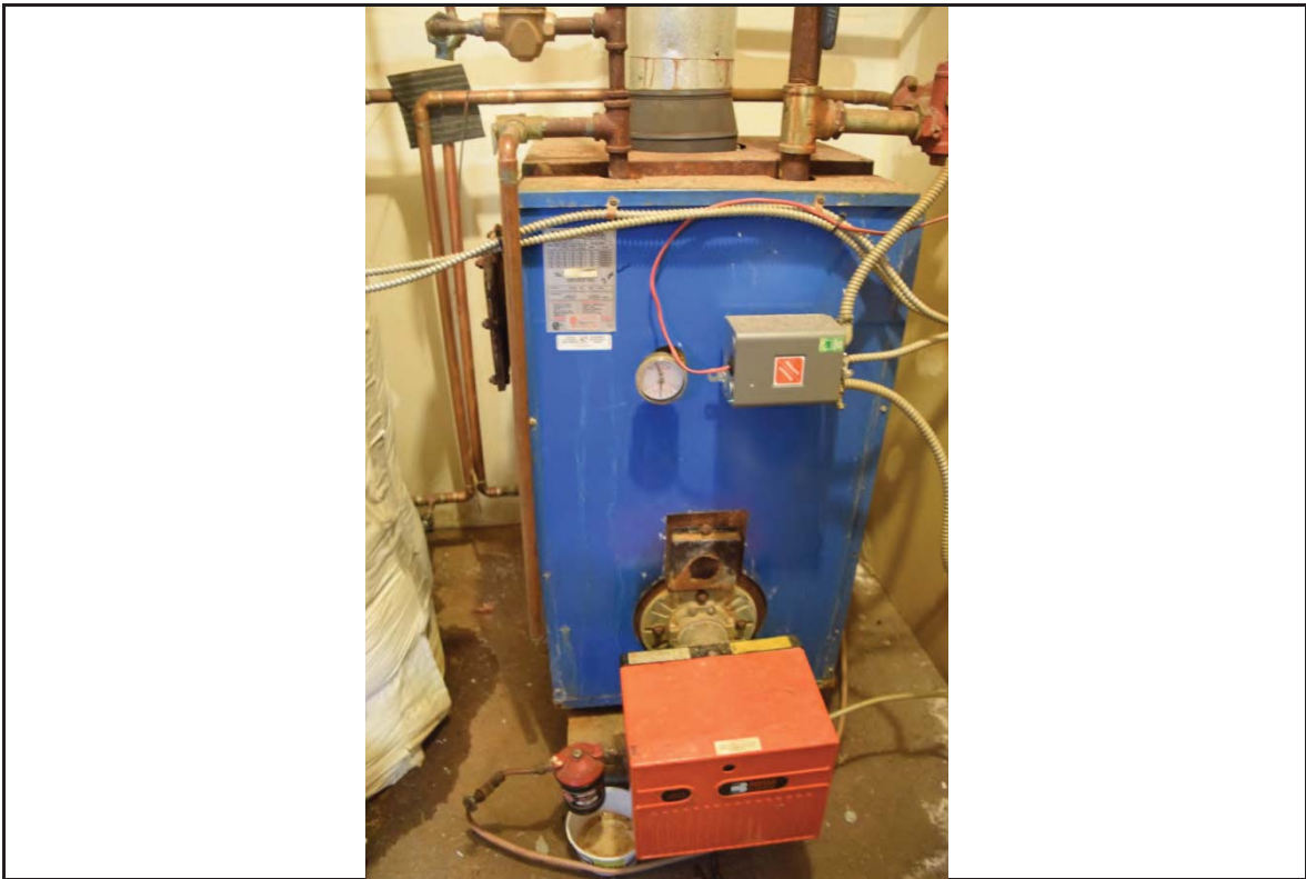
Photo 26: NY Thermal Boiler
