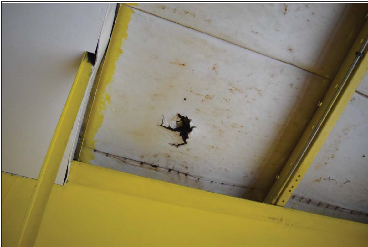
Photo 22: Typical Tear in Roof Insulation Membrane
