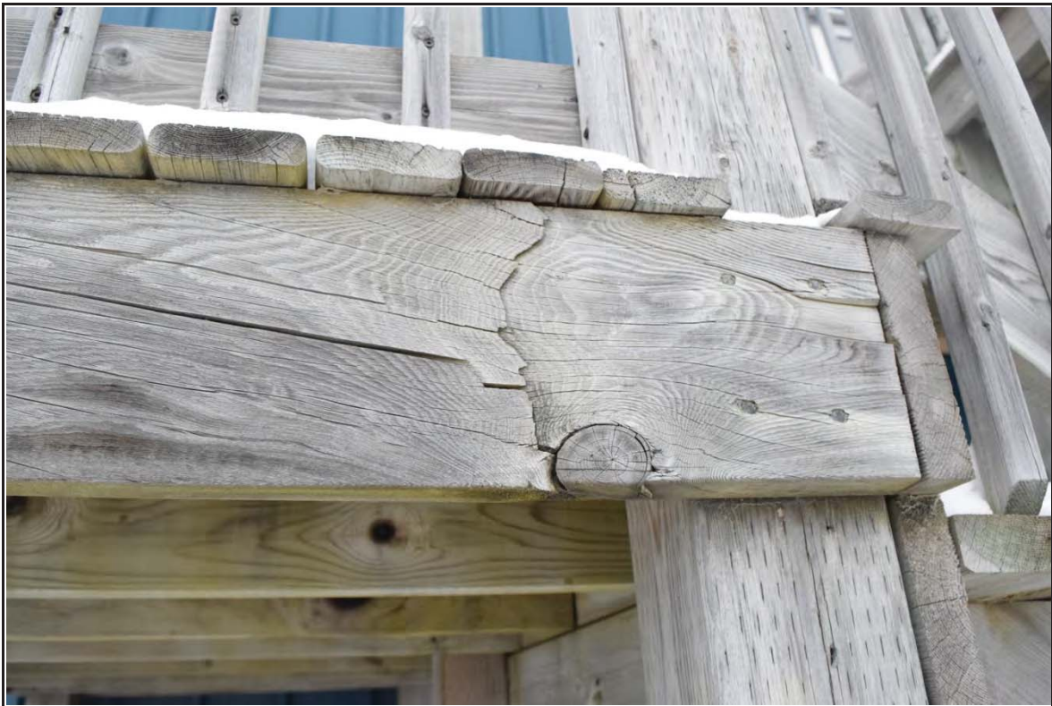
Photo 10: Cracking to Wood Stair Rim Joist
