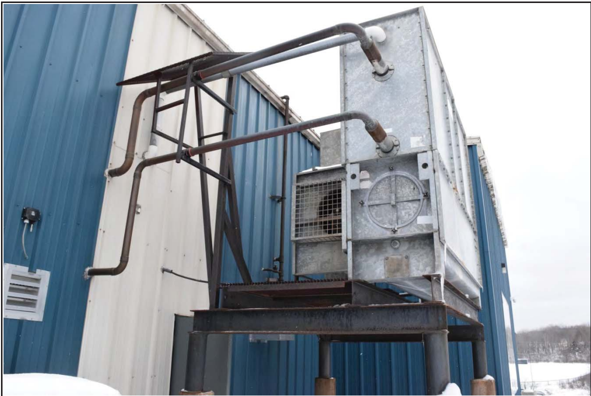
Photo 38: Ice Plant Condenser
