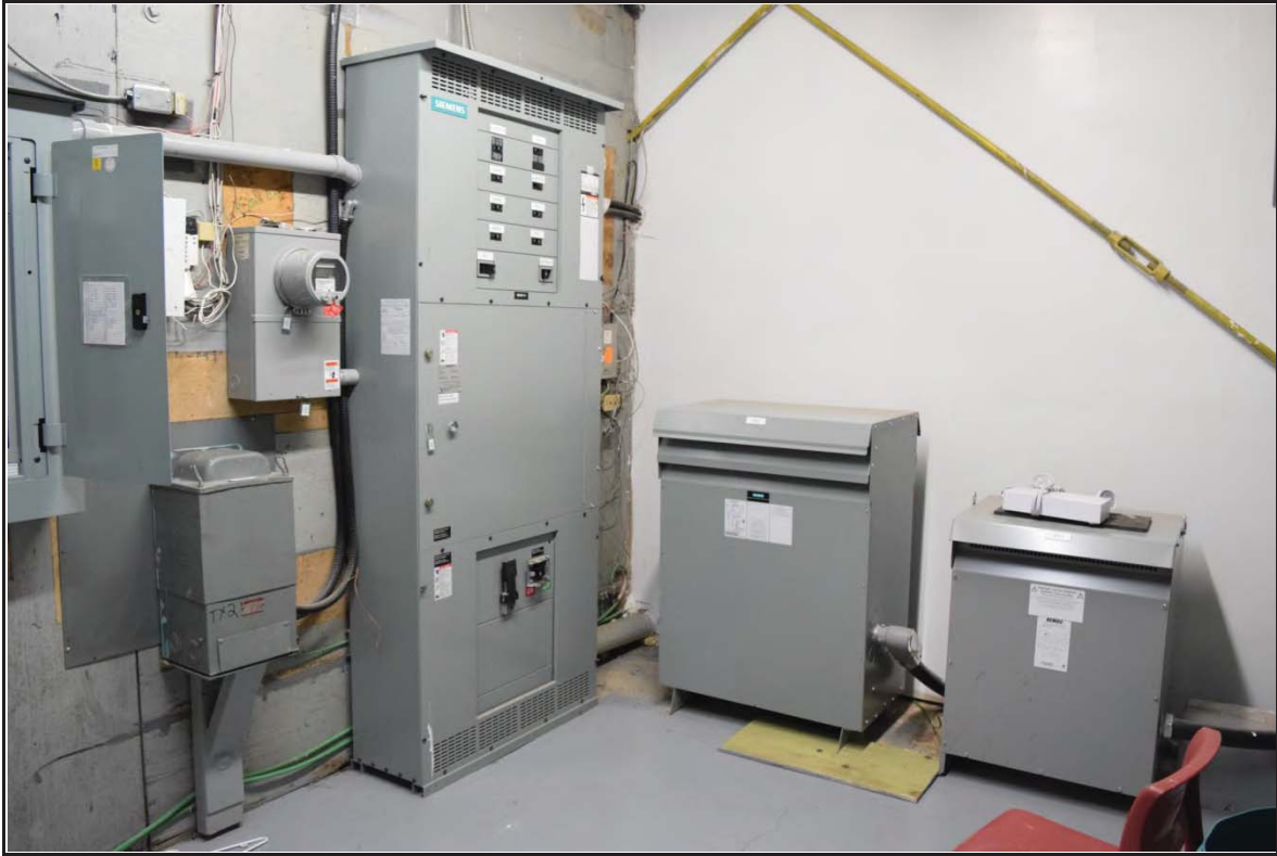
Photo 31: Main 800A 347/600 Disconnect, Distribution, and Transformers
