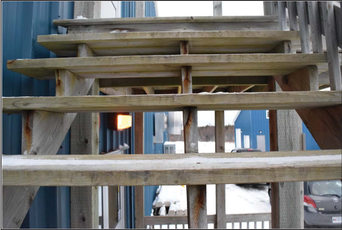
Photo 11: Deterioration to Wood Stair Stringers
