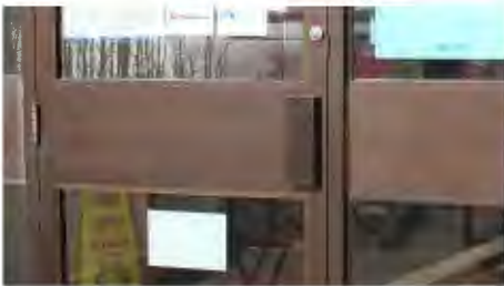
MB 22 | Entrance Door Hardware
