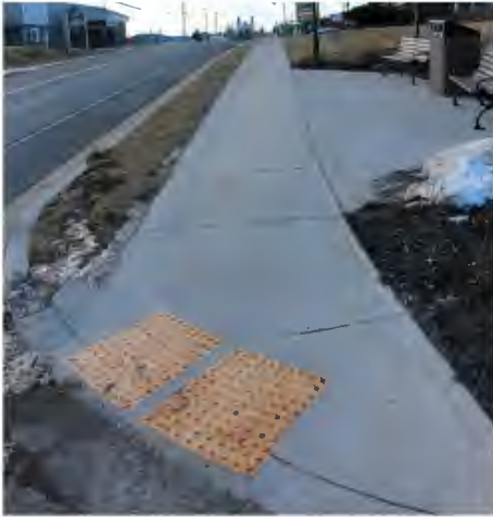
MS 1 | TWSI at end of sidewalk along with a rest area for pedestrians
