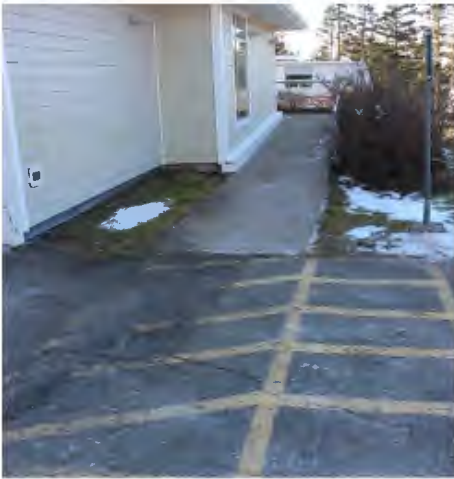
MB 12 | Accessible Ramp Landing
