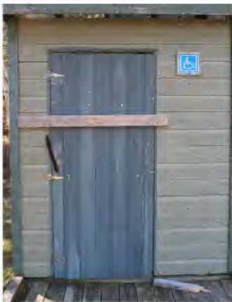
PA 4 | Accessible Washroom
