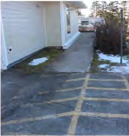
MB 12 | Accessible Ramp Landing
