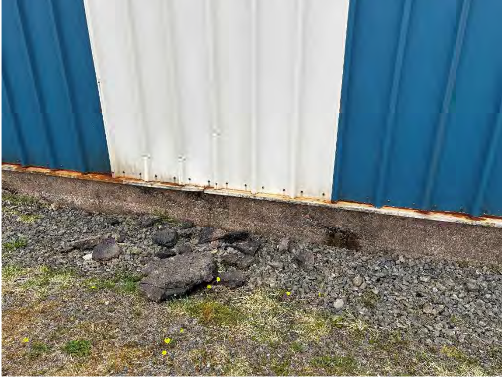
Photo 9 – Corroded Metal Siding and Foundation on North Wall.
