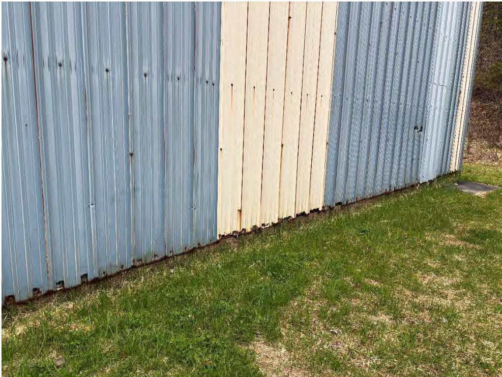
Photo 10 – Corroded Metal Siding and Foundation on South Wall.
