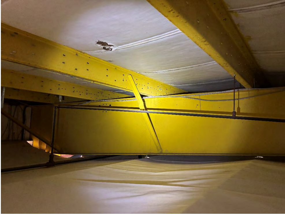
Photo 13 – Diagonal Flange Brace Damaged Possibly by Buckling.
