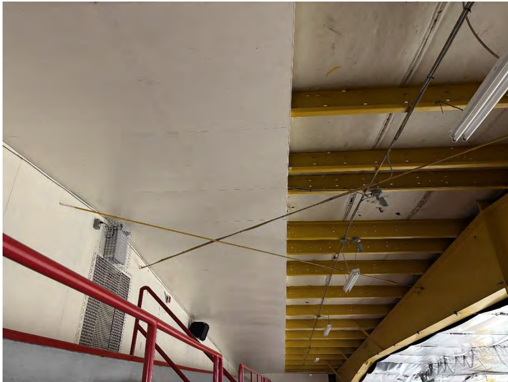
Photo 6 – Misaligned Lateral Rod Roof Bracing in Last Bay at East End of Building.
