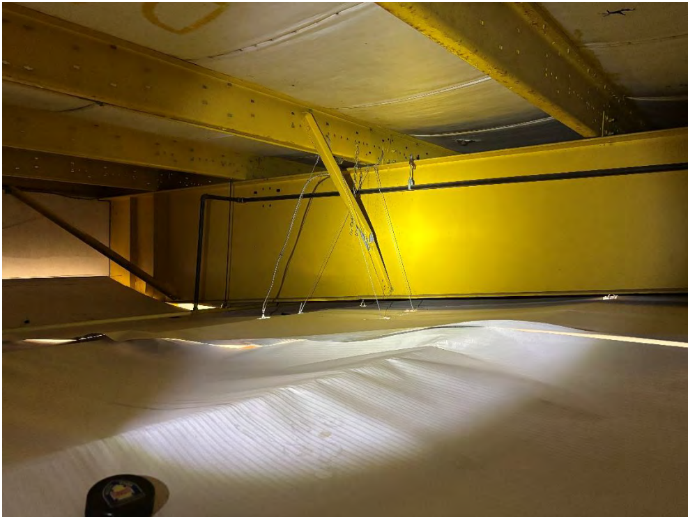
Photo 12 – Diagonal Flange Brace Damaged by Impact.
