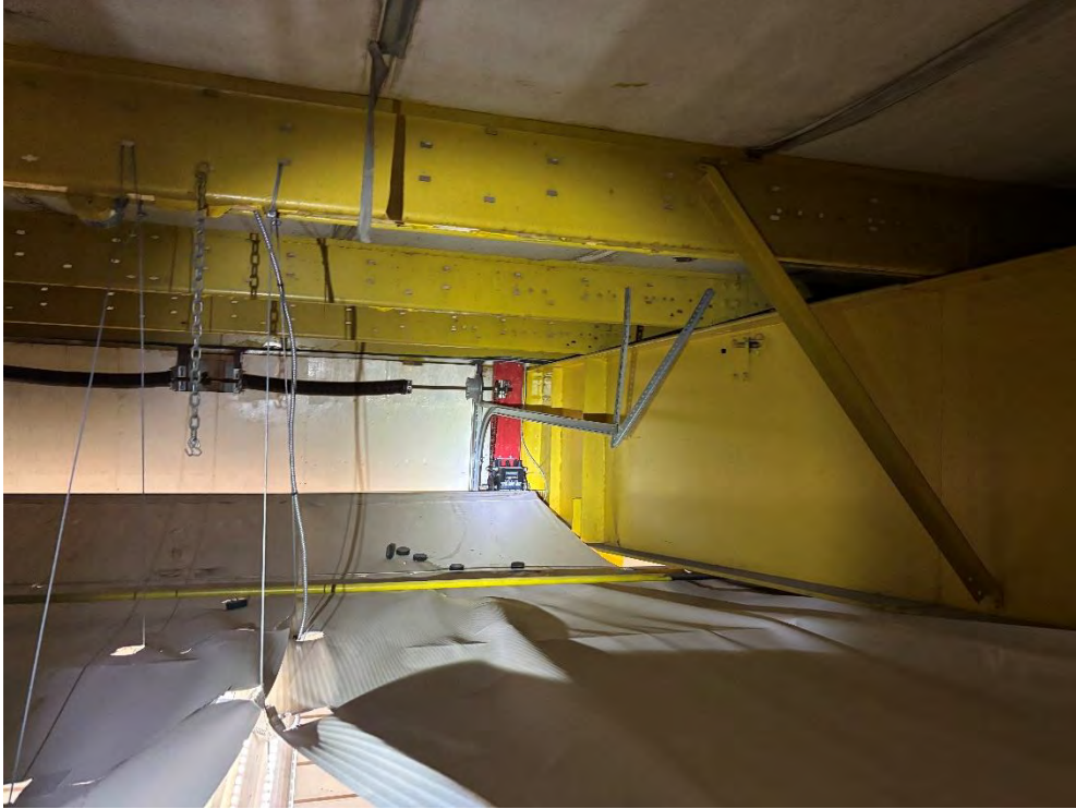
Photo 11 – Diagonal Flange Brace Removed due to Interference with Overhead Door Track.
