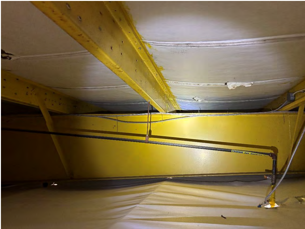
Photo 14 – Gap Between Purlin and Clip Indicates Purlin Rolling.
