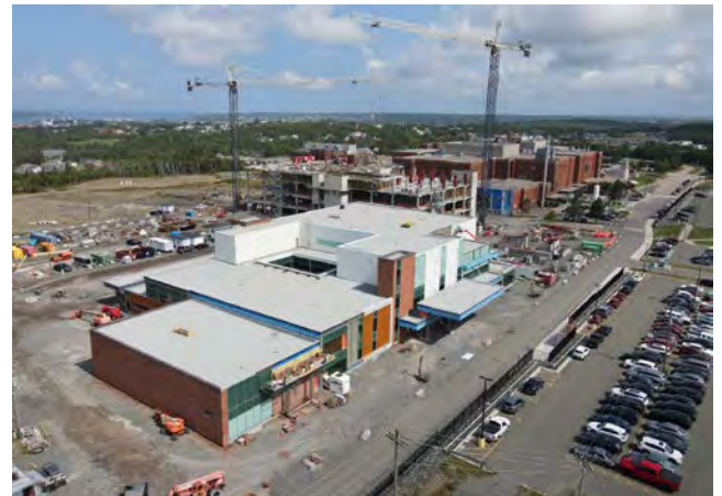
Aerial shot of the new Cape Breton Cancer Centre, behind Cape Breton Regional Hospital, showing ongoing construction.
